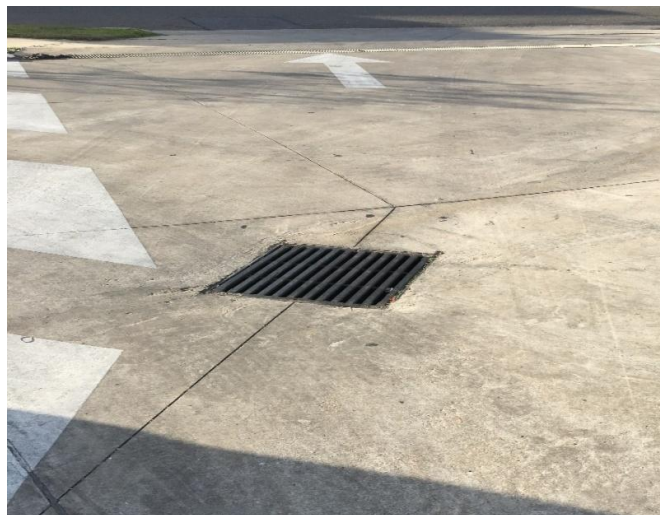
Figure 2: Image of Storm water collecting system in the service station
