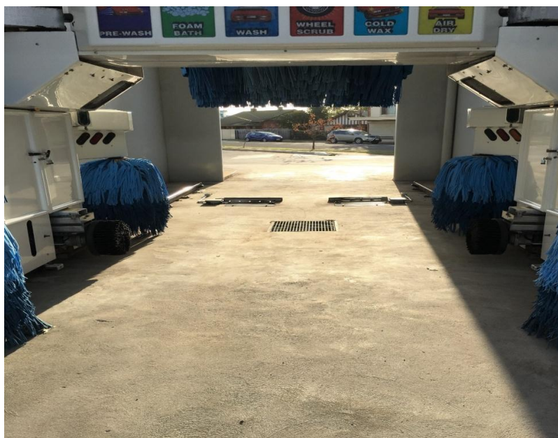
Figure 4: Image of car wash system in a service station
